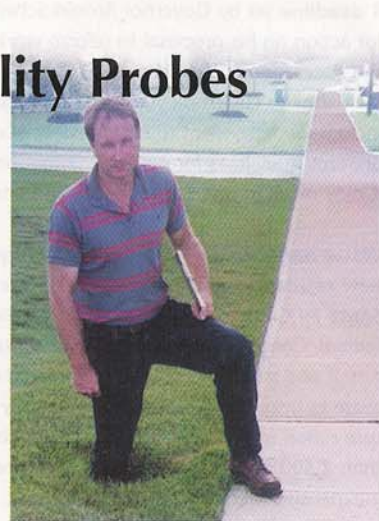
Engineer Michael Pierce stands knee-deep in a sinkhole in this photo, which ran in a number of newspapers after it was displayed at hearings held by New Jersey state investigators. The cause was traced to an unconnected drain pipe joint, which Pierce believes was overlooked by town inspectors.
